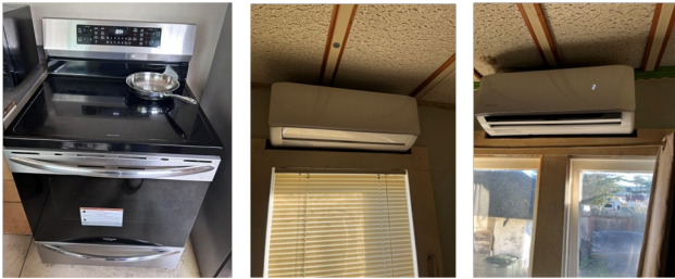
Figure 12: Kim Residence with Upgraded Induction Range and Ductless Mini Split
