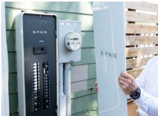
Figure 5: Span.IO Smart Panel
