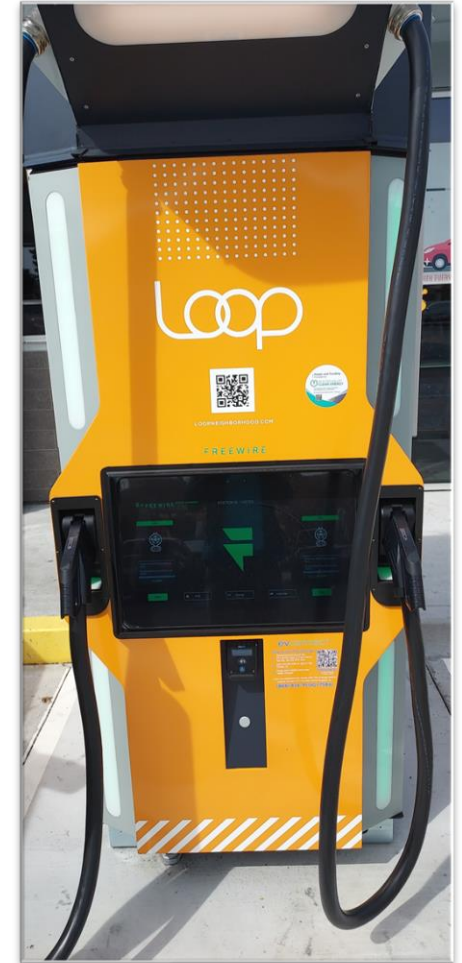
Dual port charger (200 kW) with integrated battery storage in Mountain View
